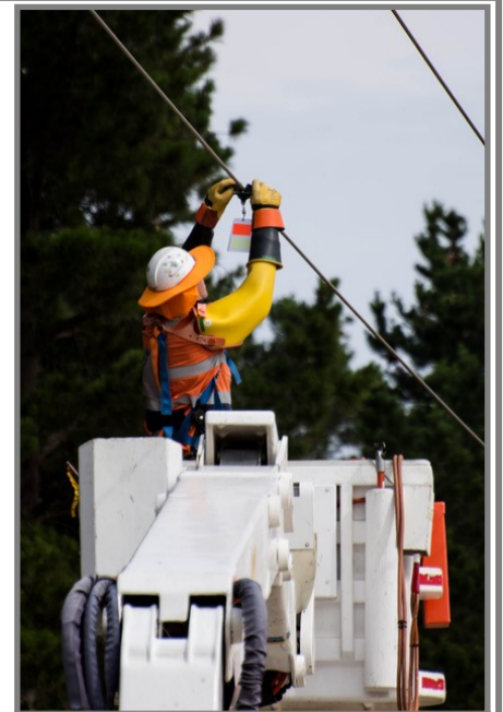
Bird flapper discs being installed on a powerline by TasNetworks Photo supplied
