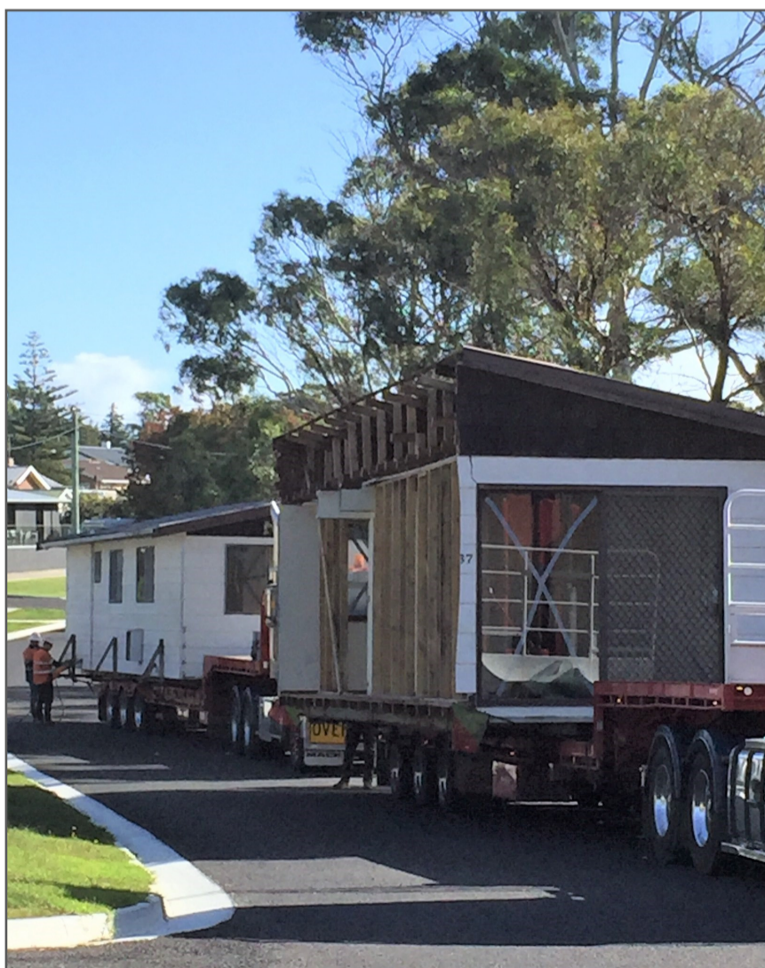
Moving house, literally! This house in Bentley St recently was neatly cut in half, loaded onto a low loader and moved off to reside somewhere else.
